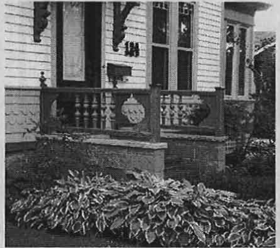
The railing of this new porch is made of traditional elements, but they are not arranged in a typical pattern. The brackets are also traditional, but perhaps too large for the application. Concrete block is not an appropriate material for a house of this type. (See "Preserving Porches.")
