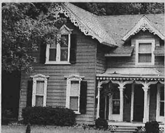
The details on this house are well preserved, with the exception of the added wood shutters.
