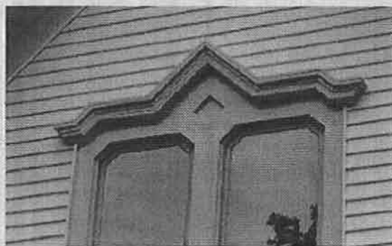
Inappropriate enclosure of historic wood trim with aluminum.
