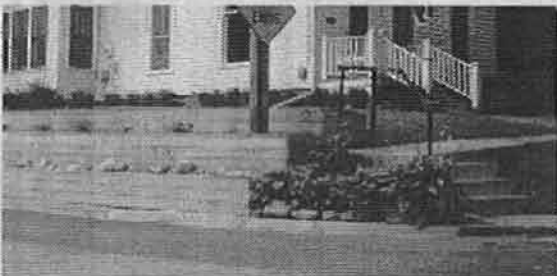
Inappropriate railroad tie retaining wall.
