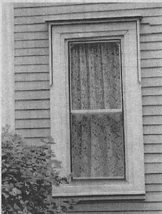
Inappropriate reduction of historic window opening to fit standard sized replacement window. ("Panning")
