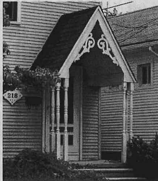
The wood columns are structurally capable of supporting this roof, but they are not in proportion. They are too thin for their height. (The use of spindles instead of columns is not a historically accurate detail.)
