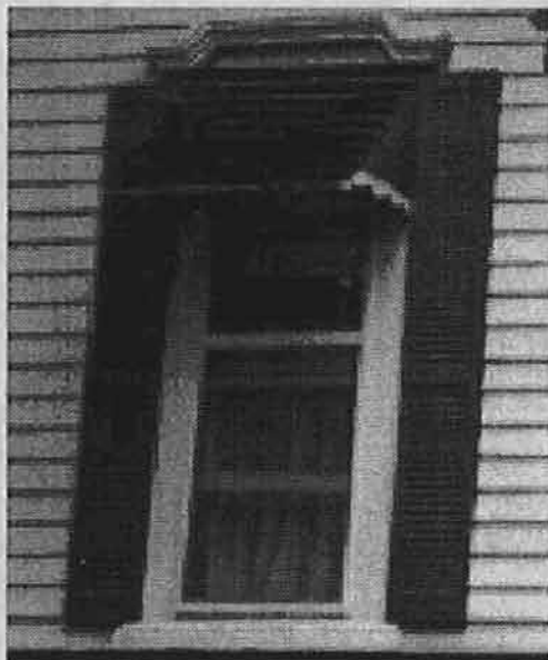
The metal awning and inoperable shutters are not historically appropriate window treatments. The awning also obscures the original window hood trim.
