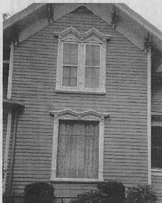
Inappropriate replacement window on first floor. The dividing mullion and historic casing have been cut and a non-historic picture window inserted.
